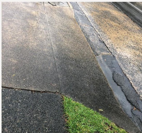
Figure 4 - View of the existing crossover on Homer Street at the front of the subject land
