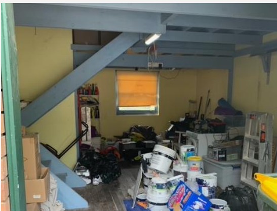
Figure 7 – View north inside the existing garage showing wooden floor and mezzanine to be demolished.
